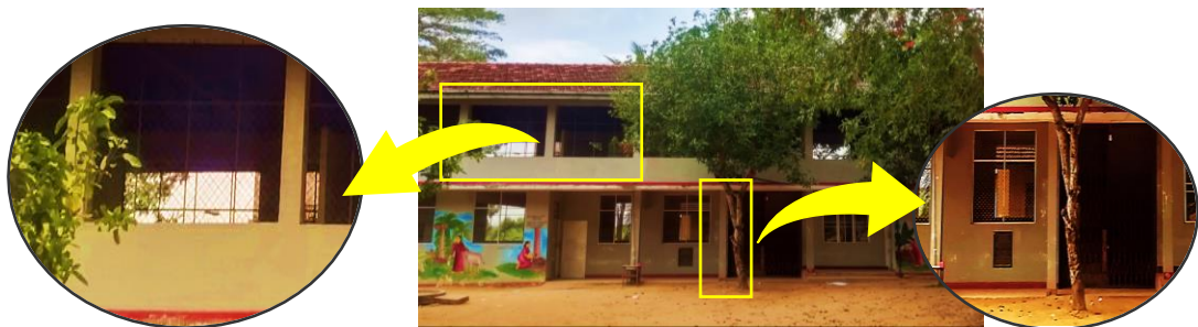
Figure 7-7. Short column effect in school buildings
