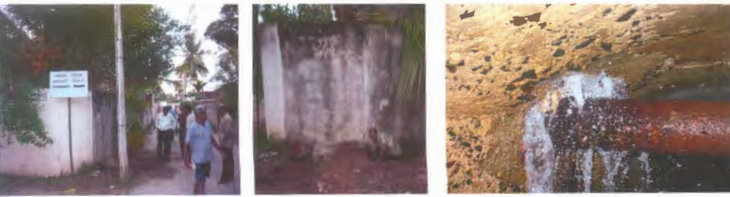
Figure 4-26 Culvert Crossing Leak Investigation in two roads
