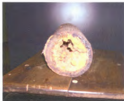
Figure 1-9: Status of smaller diameter pipes in Colombo distribution system
