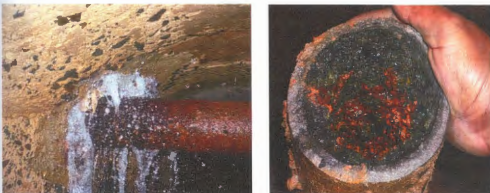
Figure 4-2 : Leaking Cast Iron pipe and Scaled Cast Iron pipe
