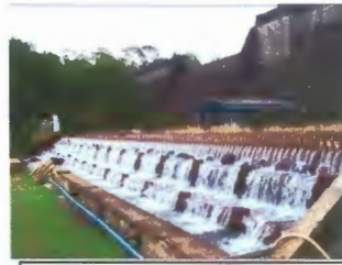
Kalatuwawa Treatment Plant
