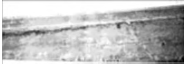
Figure. 3.6. Failures in pavement and walls
