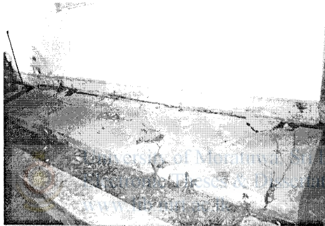
Figure 3.7 Failures in pavement
