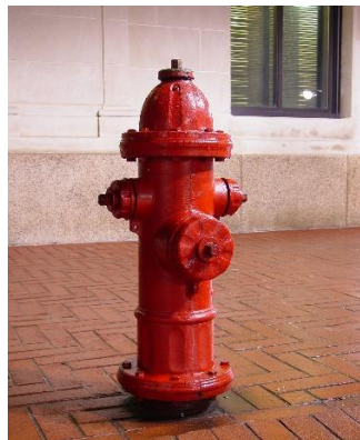
Figure 29: External fire hydrant
