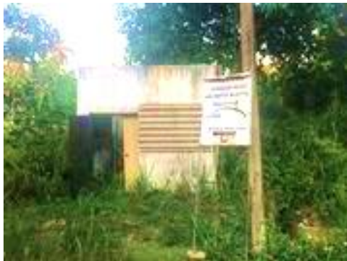
Figure 49: BH P - Abandoned incinerator in unsafe conditions
