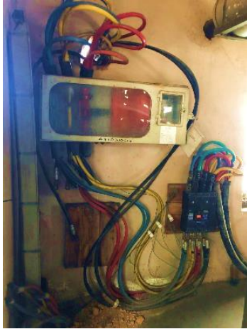
Figure 52: DGH S - Electrical wiring in unsafe conditions
