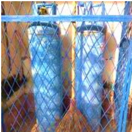
Figure 53: DH Q - Flammable materials stored next to kitchen gas
