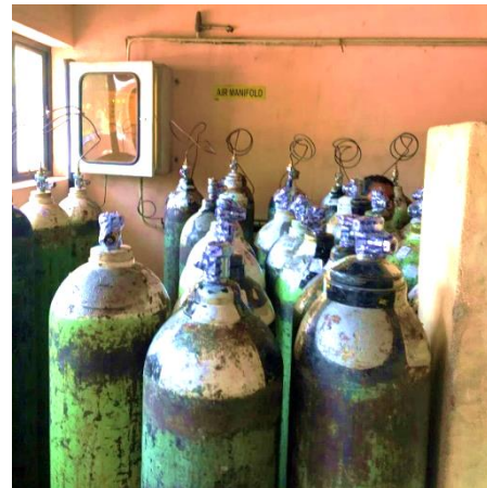
Figure 55: BH U - Safe storage of medical gas
