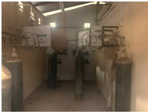
Figure 48: BH P - Manifold room in safe conditions
