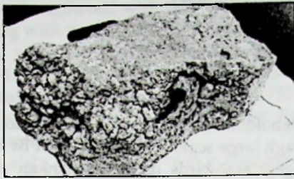
Figure 1: Deteriorated Concrete Paving Block found in Kalawila Area
