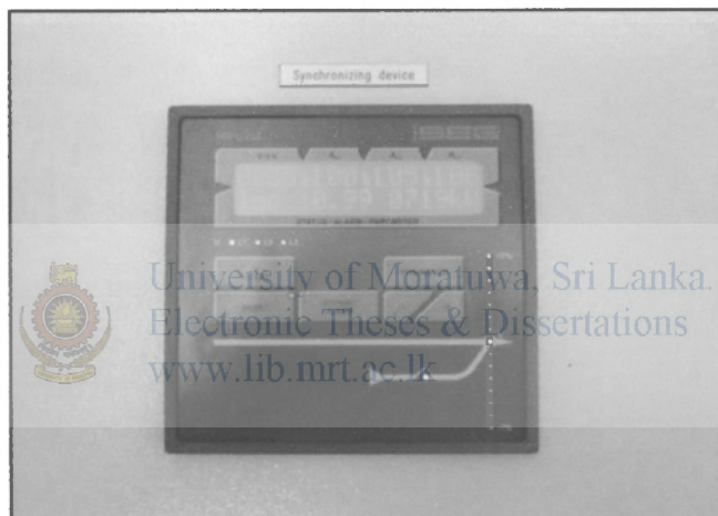
Figure 3.7 – A picture of the Automatic Synchronizer of the plant
