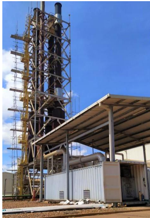
Figure 2:Installed incinerator at UJPS (Original in colour)
