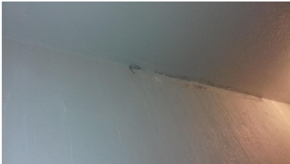
Figure 4-46: Water seepage from construction joint line at slab level of 7 th floor -
