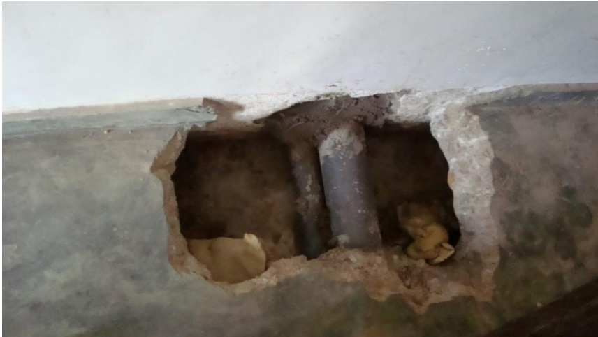
Figure 4-7: Deteriorated surface of Goda canteen rooftop - 5
