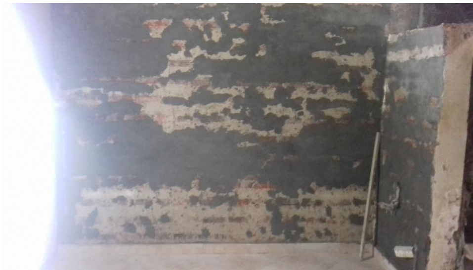
Figure 4-22: Initial surface with the deteriorated plaster chipped off and catch up plaster applied
