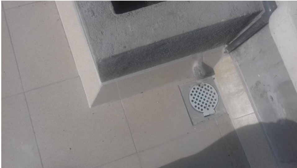
Figure 4-61: Rooftop drainpipes to facilitate proper drainage
