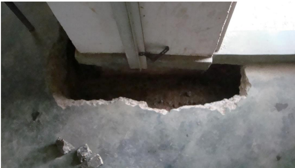
Figure 4-3: Deteriorated surface of Goda Canteen rooftop - 1
