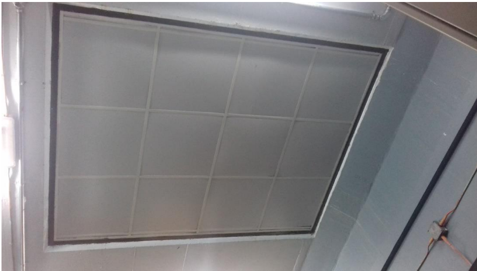
Figure 4-66: Bottom surface through which water leaks in
