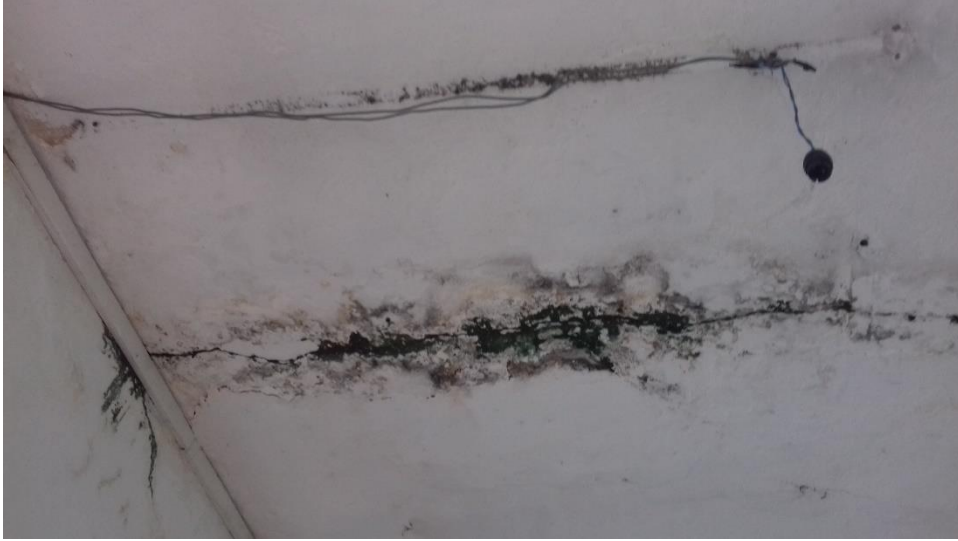
Figure 4-77: Structural deterioration of ground floor slab level due to lack of waterproofing - 1
