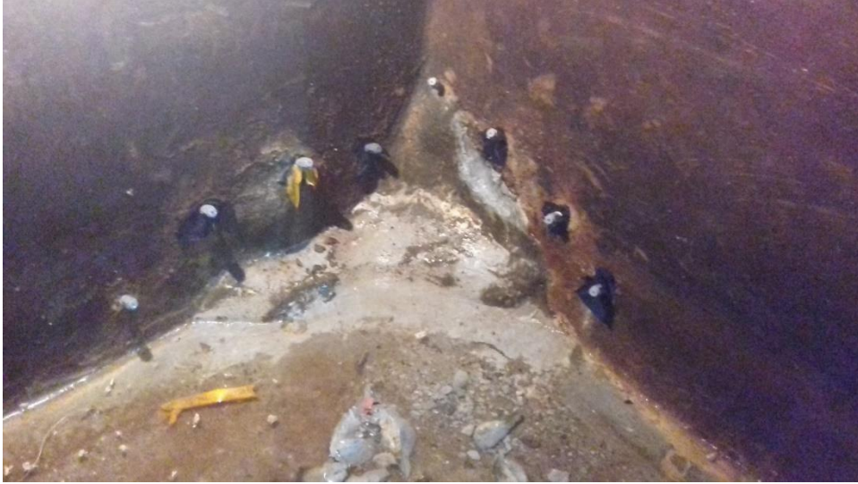
Figure 4-38: Non-return nozzles fixed to inside walls for the injection process - 1 During this injecting process, the injected product seeps out from another location. Care must be taken here to be on the lookout for such.
