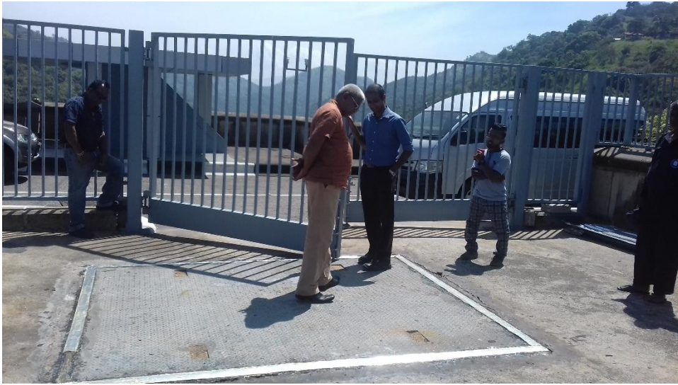
Figure 4-65: Top surface of the underground control room from which water leaks in
