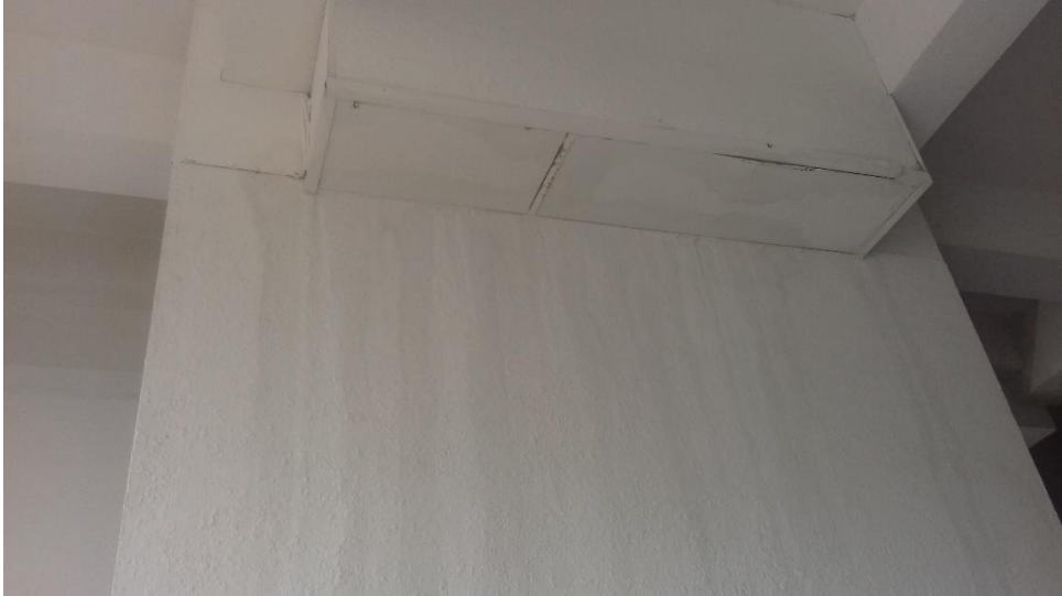
Figure 4-50: Water seepage along the walls from the duct line in the ground floor
