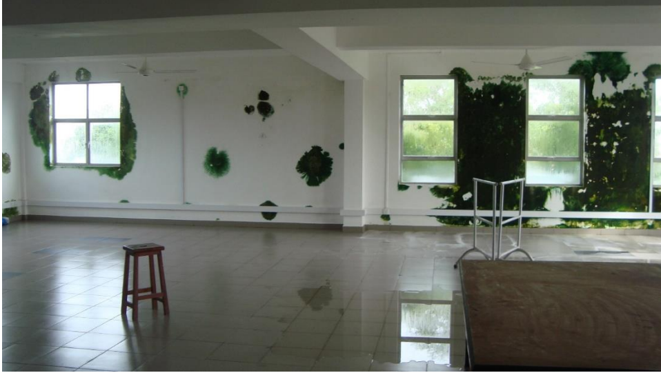
Figure 4-15: Deteriorated surface of the new building of the Textile Engineering department - 5
