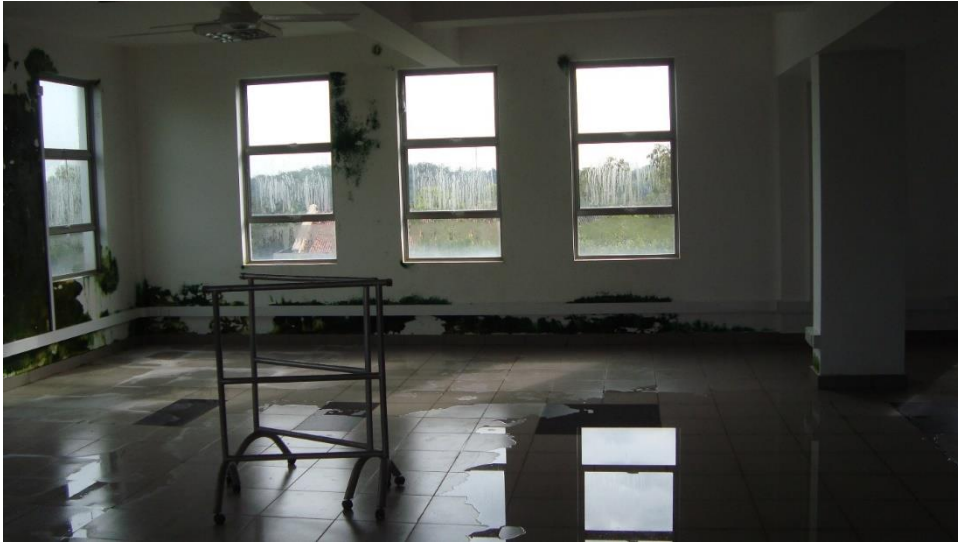
Figure 4-16: Deteriorated surface of the new building of the Textile Engineering department - 6
