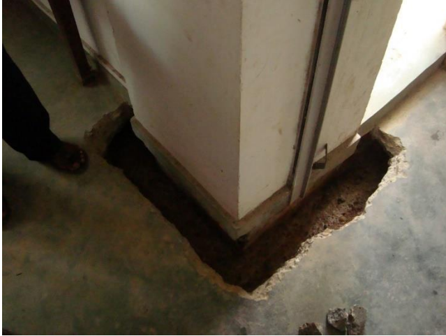
Figure 4-6: Deteriorated surface of Goda canteen rooftop - 4
