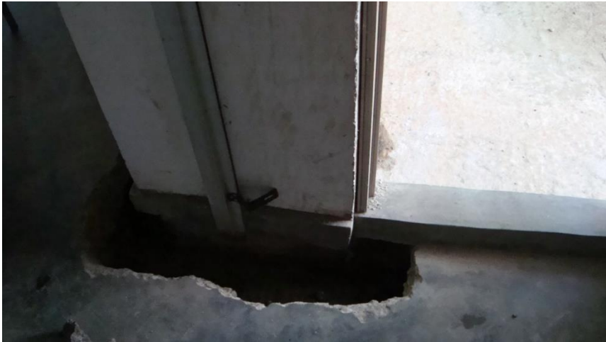
Figure 4-5: Deteriorated surface of Goda canteen rooftop - 3
