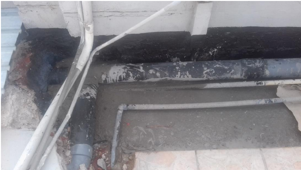
Figure 4-54: Rooftop location prone to collection of water - 2
