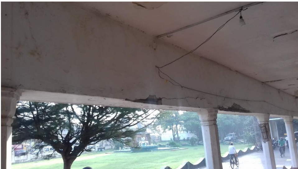
Figure 4-80: Structural deterioration of ground floor slab level due to lack of waterproofing – 4
