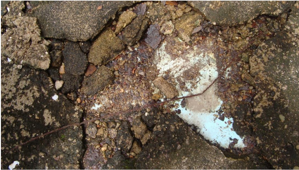
Figure 4-20: Deteriorated surface of the rooftop of the IT faculty old building - 2
