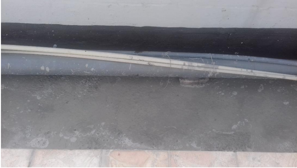
Figure 4-53: Rooftop location prone to collection of water - 1
