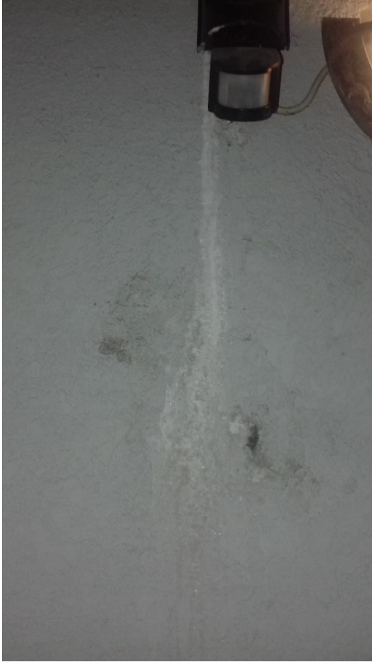
Figure 4-49: Water seepage along the wall of the ground floor
