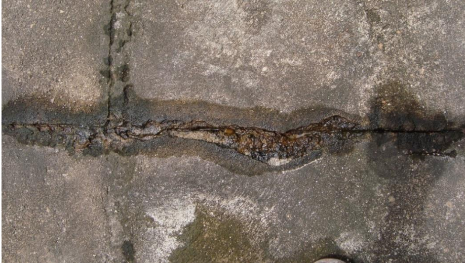
Figure 4-19: Deteriorated surface of the rooftop of the IT faculty old building - 1
