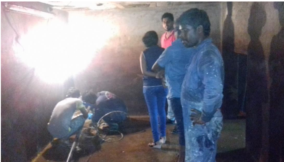
Figure 4-37: The basement of the Civil Engineering Department building prone to flooding
