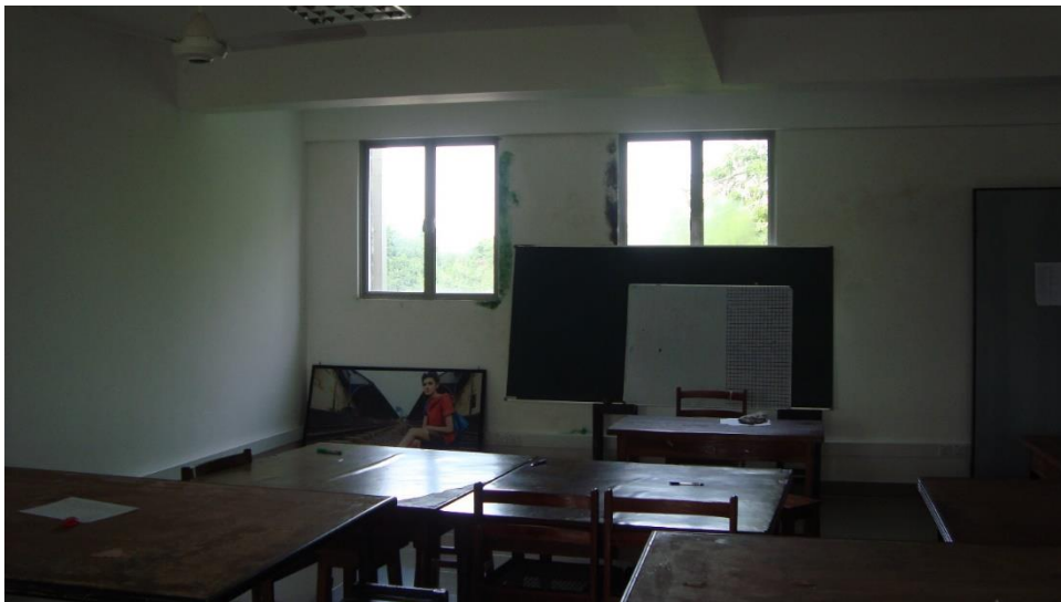
Figure 4-18: Deteriorated surface of the new building of the Textile Engineering department - 8
