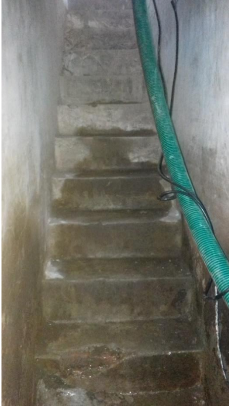
Figure 4-34: Flooding of the basement in the Civil Engineering Department building including the staircase - 2
