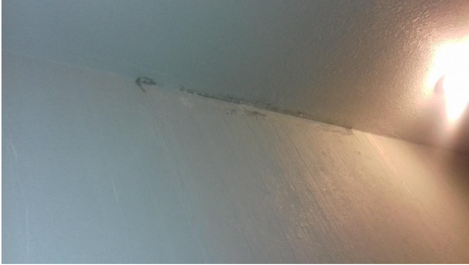
Figure 4-47: Water seepage from construction joint line at slab level of 7 th floor - 2
