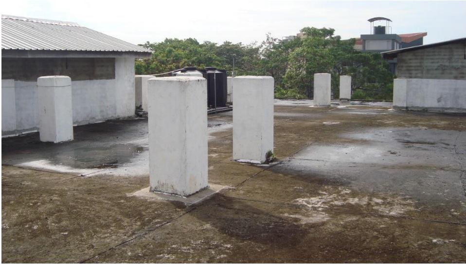
Figure 4-12: Deteriorated surface of the new building of the Textile Engineering department - 2
