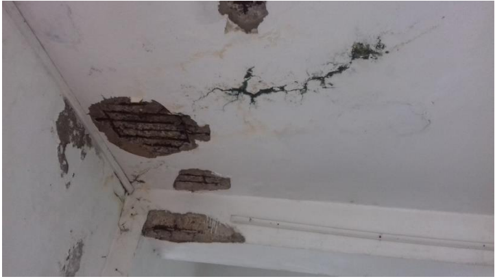
Figure 4-78: Structural deterioration of ground floor slab level due to lack of waterproofing - 2
