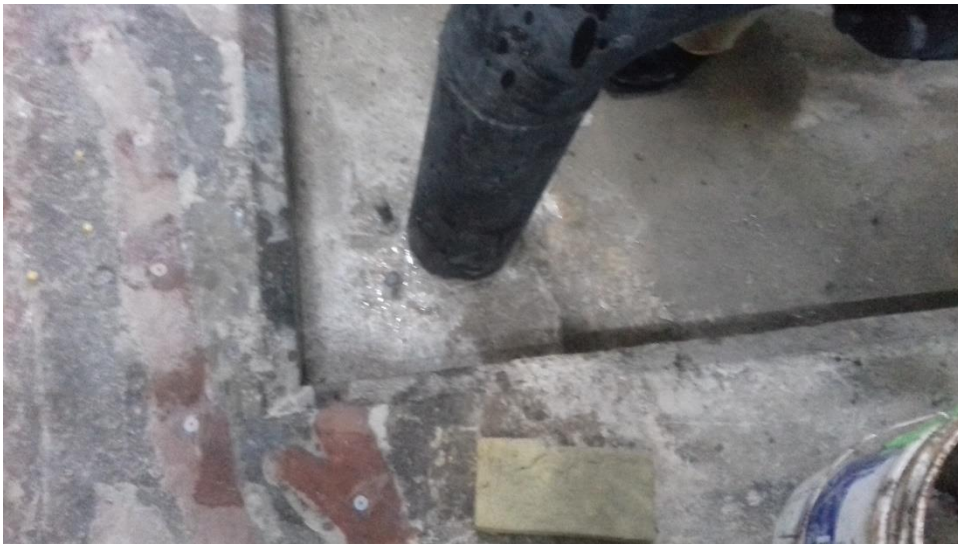
Figure 4-68: Water seeping in from puddle collar - 2
