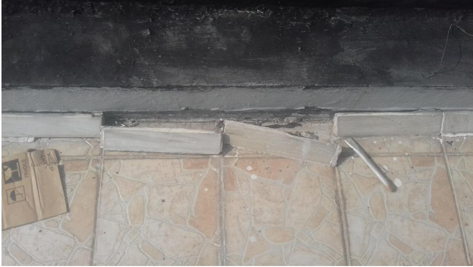
Figure 4-51: Rooftop deteriorated tile skirting expelled
