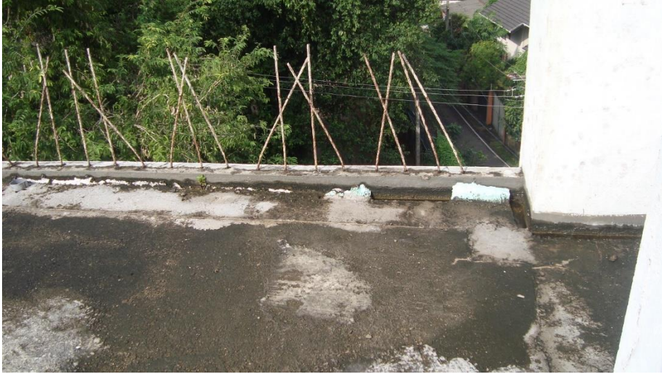
Figure 4-11: Deteriorated surface of the new building of the Textile Engineering department - 1
