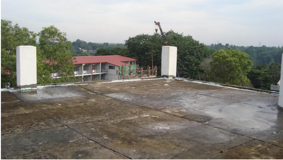
Figure 4-13: Deteriorated surface of the new building of the Textile Engineering department - 3
