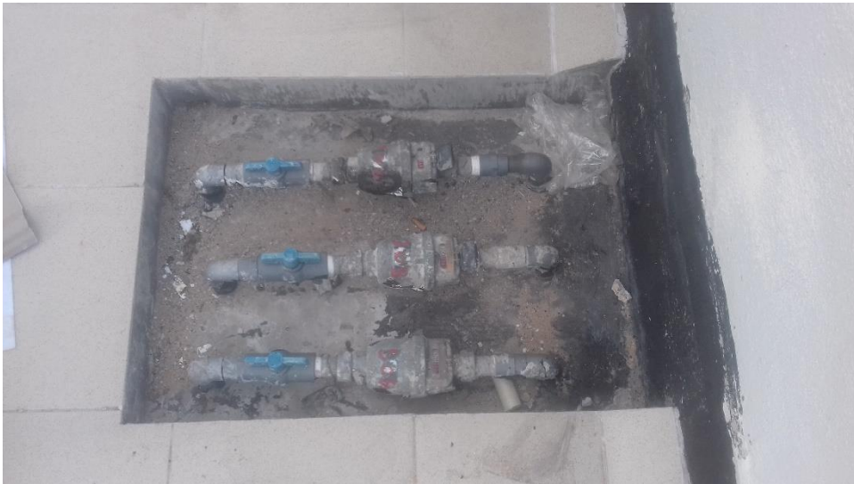
Figure 4-52: Rooftop location of water meters prone to collection of water
