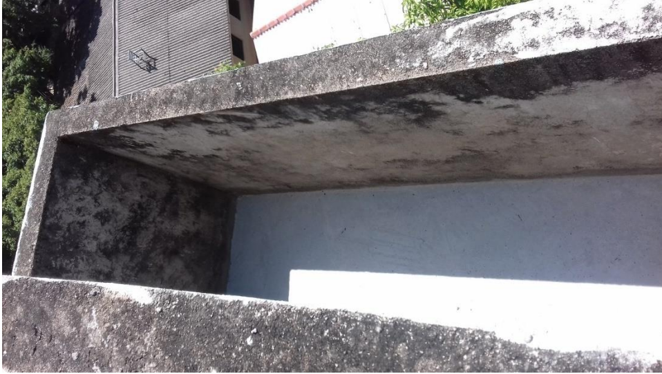
Figure 4-29: Another problematic inaccessible narrow strip of slab area
