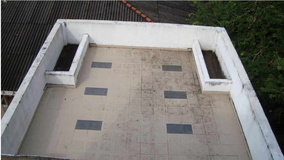
Figure 4-14: Deteriorated surface of the new building of the Textile Engineering department - 4
