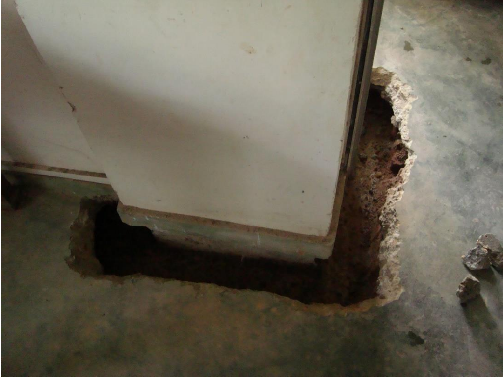
Figure 4-4: Deteriorated surface of Goda canteen rooftop - 2
