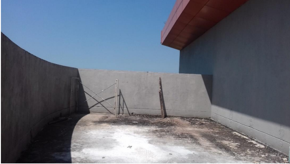
Figure 4-27: Open slab area in the IT faculty building of University of Moratuwa considered for case study II
