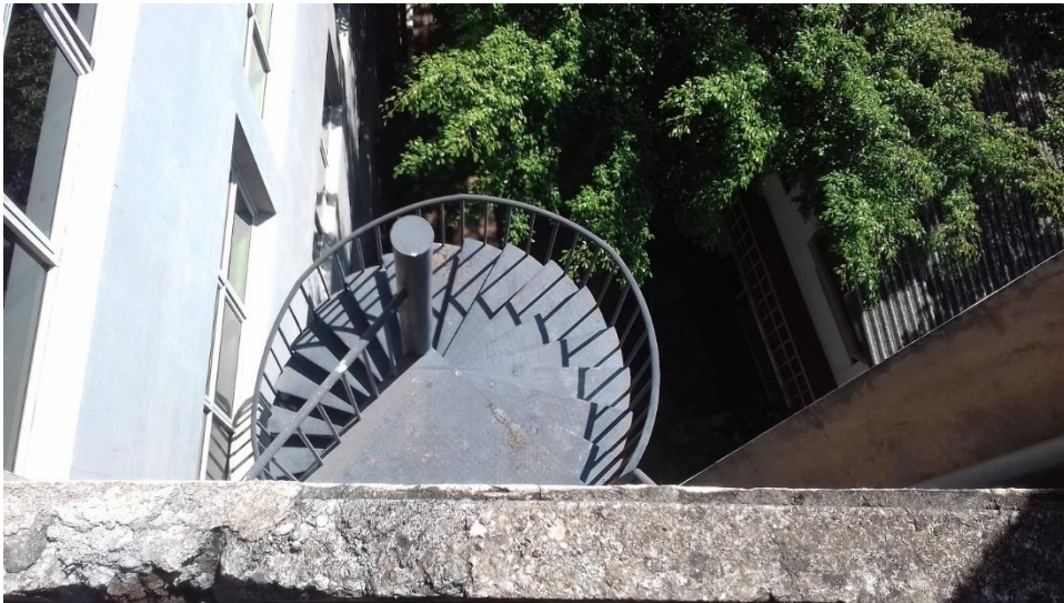
Figure 4-30: No proper means of access to the area
