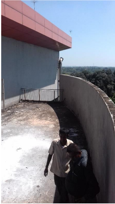
Figure 4-28: Open slab area prone to collection of rainwater
