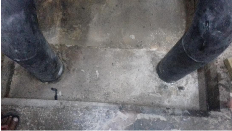
Figure 4-67: Water seeping in from puddle collar - 1
