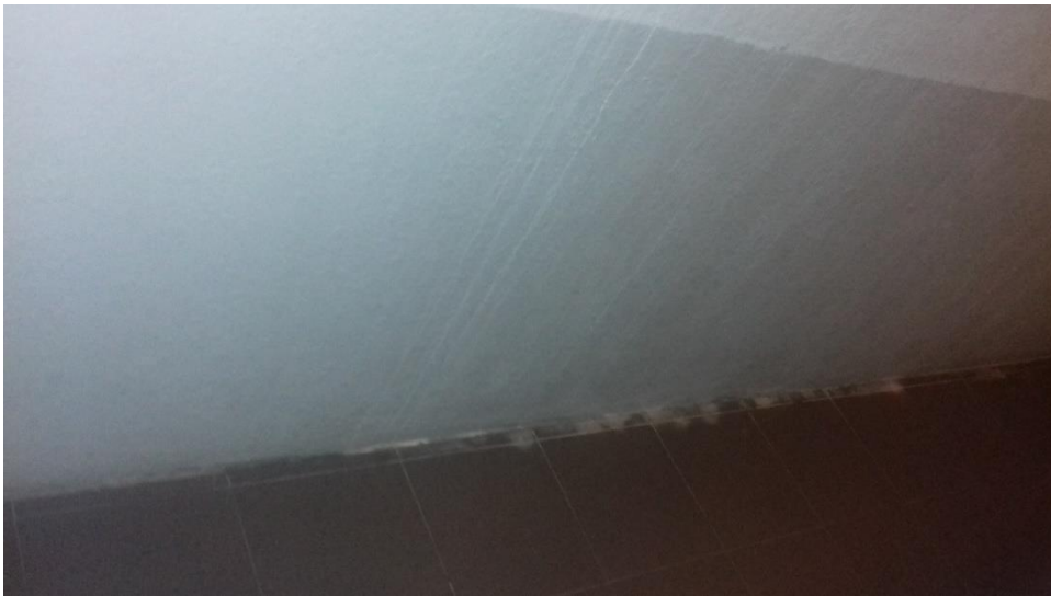
Figure 4-48: Water seepage from construction joint at floor level of 7 th floor
