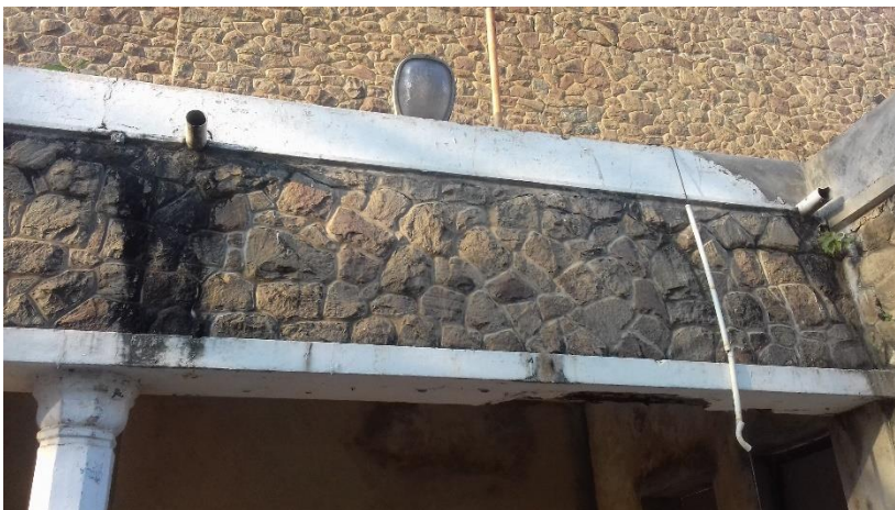
Figure 4-74: Water leaks in the front wall of the Galle Town Hall
