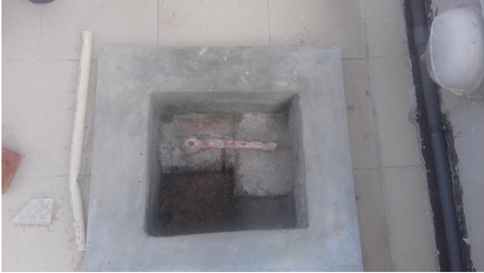
Figure 4-57: Remedial action taken to prevent collection of water at rooftop level using passive waterproofing design
