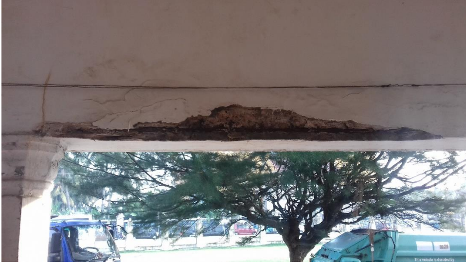
Figure 4-79: Structural deterioration of ground floor slab level due to lack of waterproofing - 3
