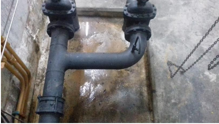
Figure 4-73: Water leaks to be injected with waterproofing solutions
