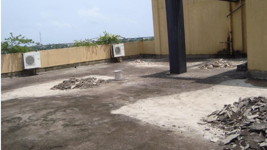
Figure 4-2: Deteriorated surface of the rooftop of the Mechanical Engineering Department new building - 2
