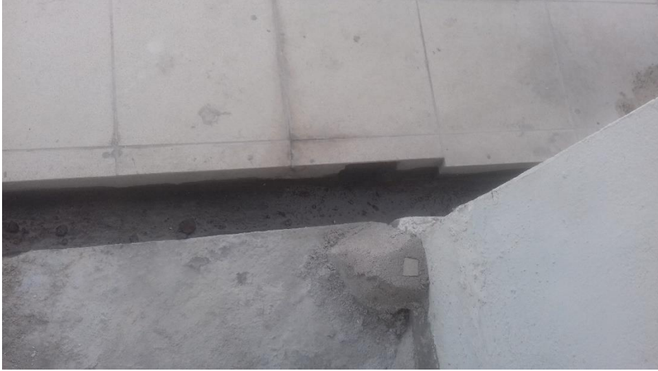
Figure 4-55: Passive waterproofing mechanism on rooftop drains into which water gets drained beneath the tile surface - 1
