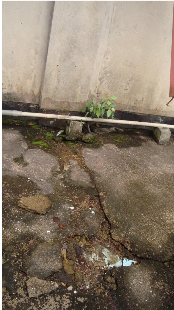
Figure 4-21: Deteriorated surface of the rooftop of the IT faculty old building - 3
