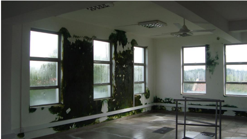
Figure 4-17: Deteriorated surface of the new building of the Textile Engineering department - 7
