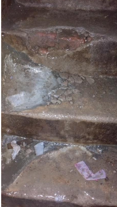
Figure 4-36: Flooding of the basement in the Civil Engineering Department building including the staircase - 4
