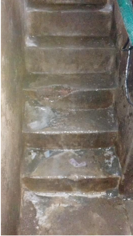
Figure 4-35: Flooding of the basement in the Civil Engineering Department building including the staircase - 3
