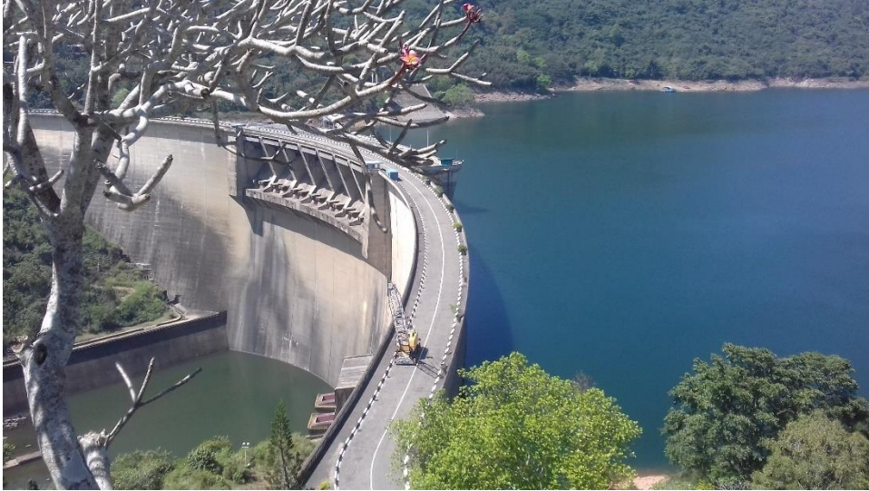
Figure 4-62: Sluice gates located at the far left were affected by waterproofing issues. The cause has been identified as a leak that sprung up due to the high pressure that the structure is being subjected to. These minor leaks were addressed by injection moulding.
