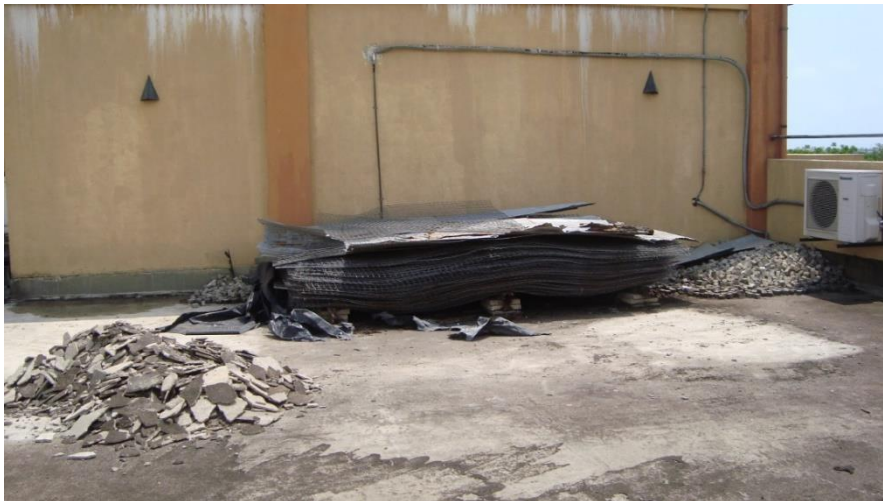
Figure 4-1: Deteriorated surface of the rooftop of the Mechanical Engineering Department new building - 1
