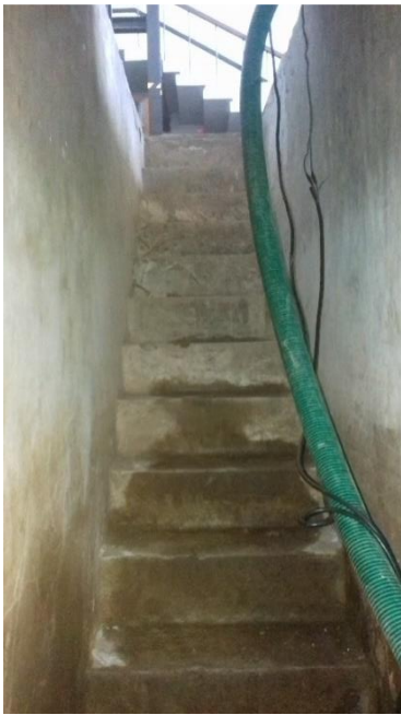
Figure 4-33: Flooding of the basement in the Civil Engineering Department building including the staircase - 1
