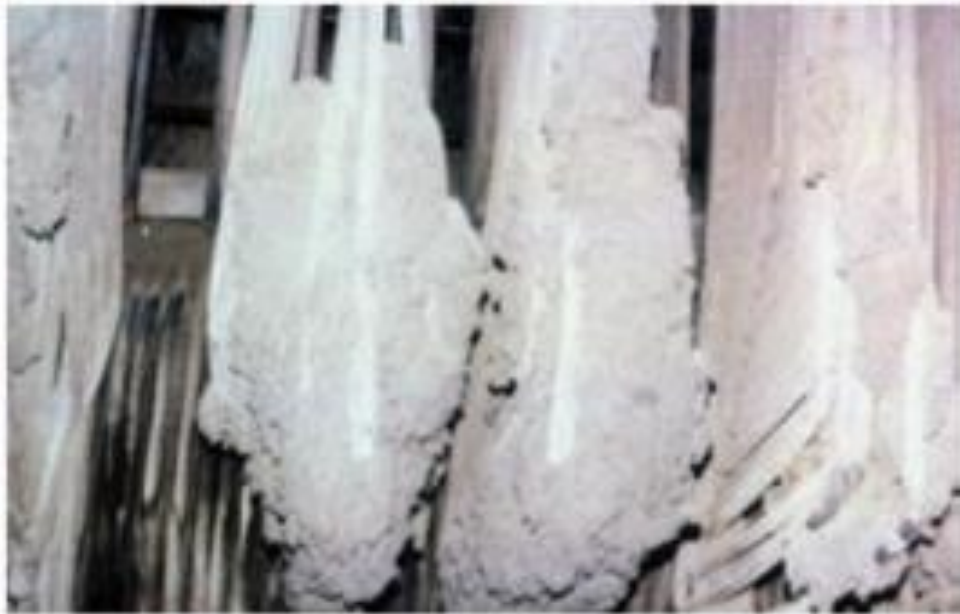
Figure 2.2: Super heater tubes
