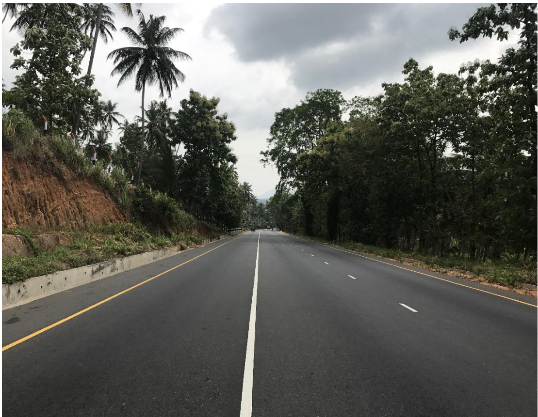
Figure 3.4 Downward view of non-corrugated pavement section (67+200 km)
