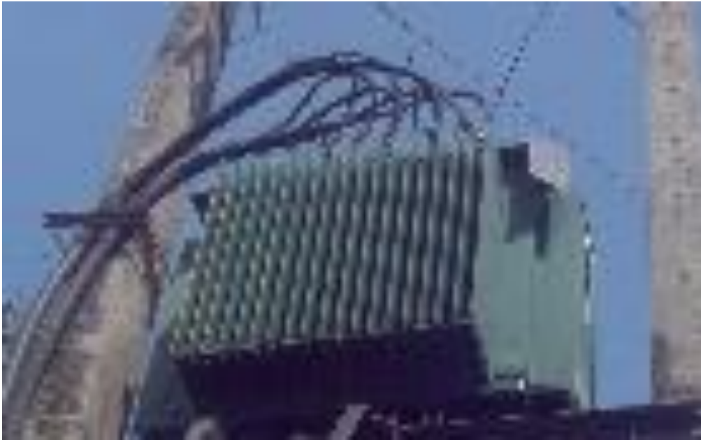
Figure 4-2 : View of the Transformer Assembly from Ground
