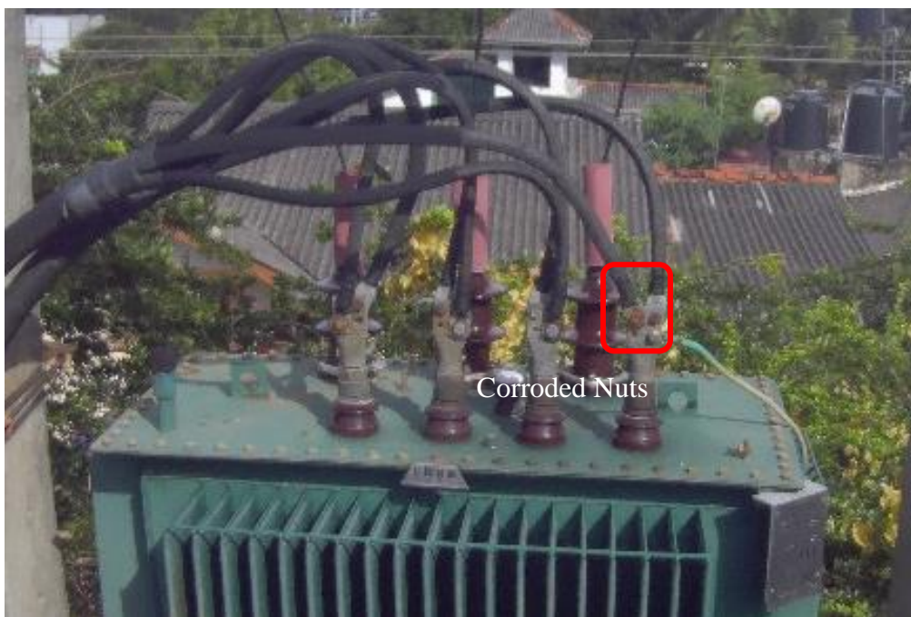
Figure 4-3 : Detailed View of the Transformer Assembly from Aerial Imaging
