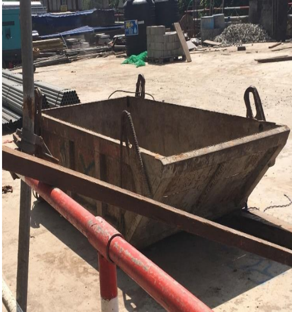
Figure 4.5: Bucket used to bring waste from upper floors to the basement in Case F
