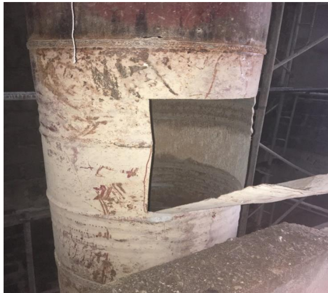
Figure 4.4: Garbage chute made out of barrels in Case E
