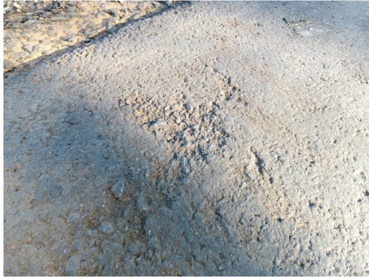
Figure 41. Segregated pavement surface
