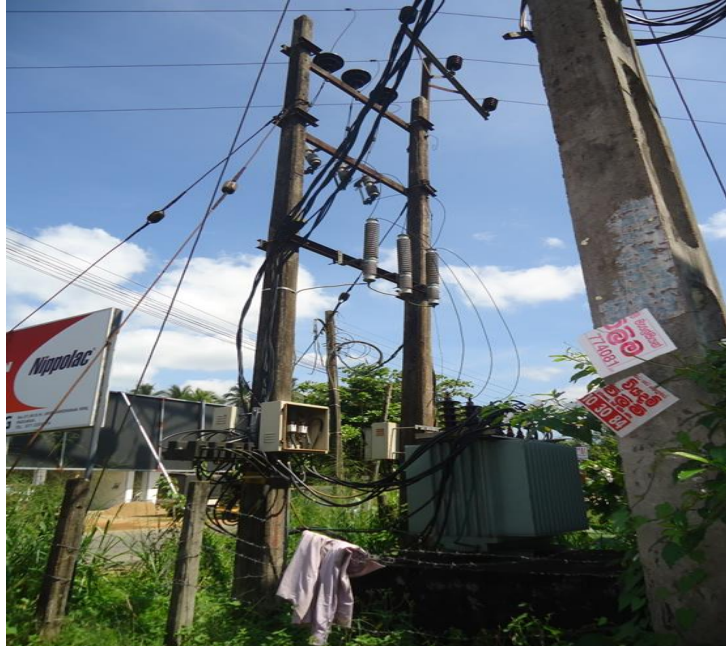
Figure 6: Negligence of workman
