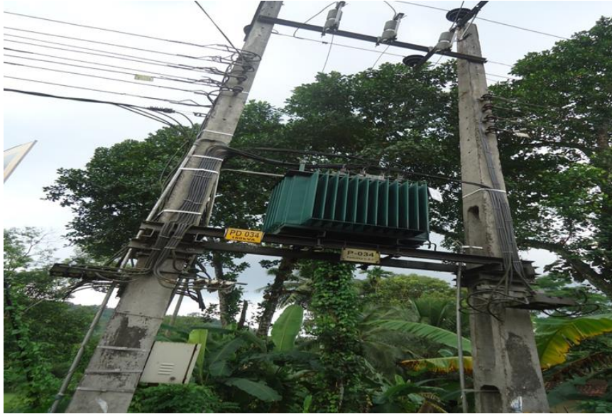
Figure 8: Neatly arranged substation
