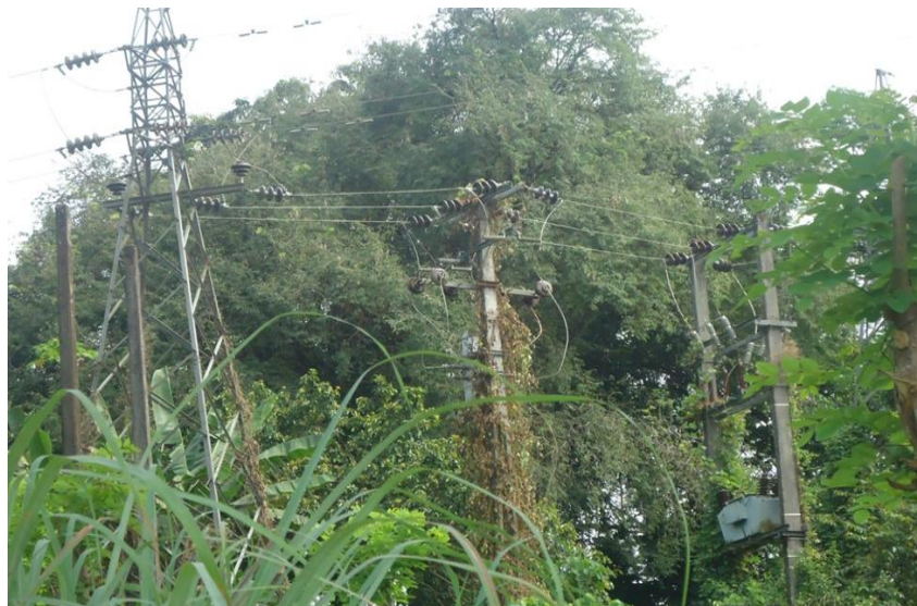
Figure 9: Abandoned power line
