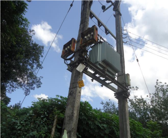
Figure 4: Damage fuse boxes
