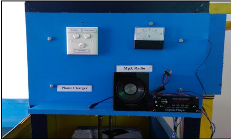
Figure 4.17: Power Distribution of the WEC
