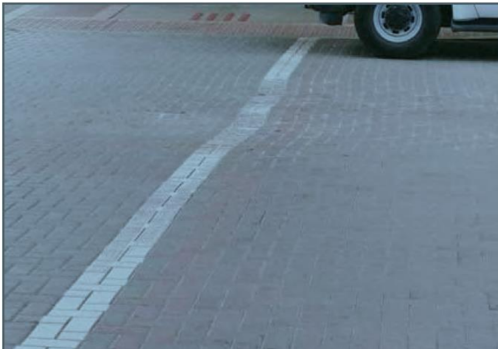
Figure 3-5 Sample distress (Low severity)
