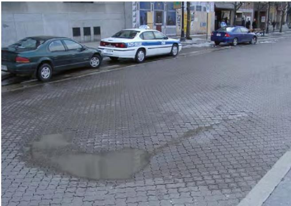
Figure 3-4 Sample distress (High severity)
