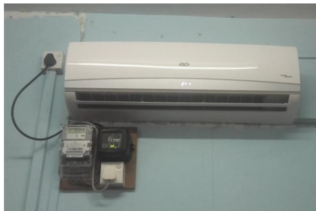
Figure 5.2: Load Controller Module
