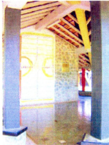
Figure 74 : Entering is creates by a grey colour entrance SOS youth village, SOS Village, Piliyandala.
