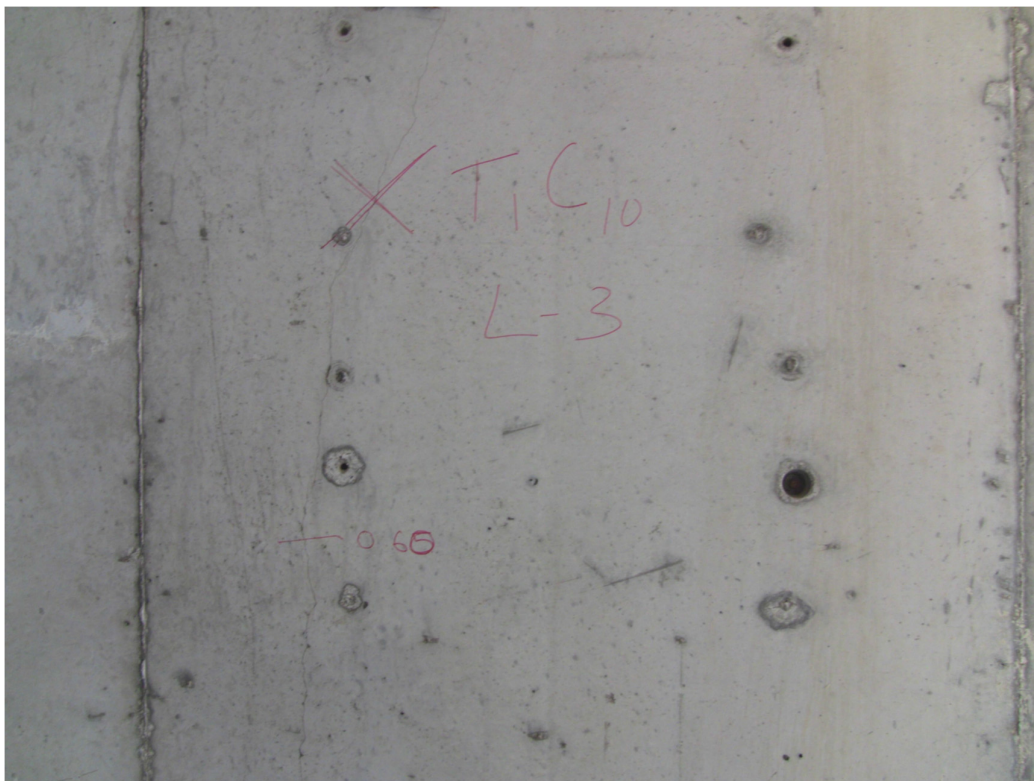
Figure 11: Vertical crack observed [Project in Colombo]
