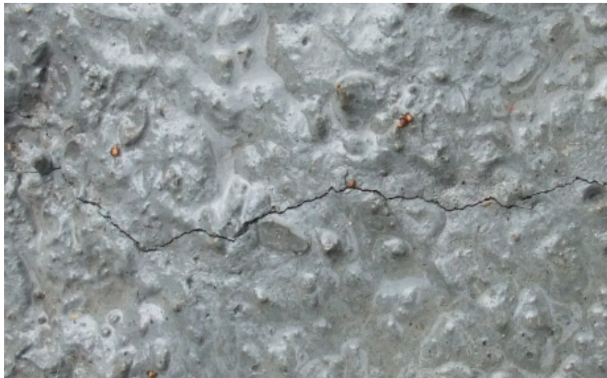
Figure 06: Chemical shrinkage cracks in concrete. [ http://www.concrete.org.uk ]
