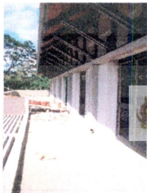
figure 3. :the roof touching the wall is not visible but create sensitive mystic quality
