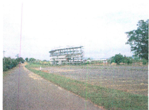
Figure3.5 : as one approaches the building it is the vertically emphasised elevation that is to be experienced. This have a proportion giving the vertical emphasis and the transparency gives the temporary nature of the place reflecting its identity. .
