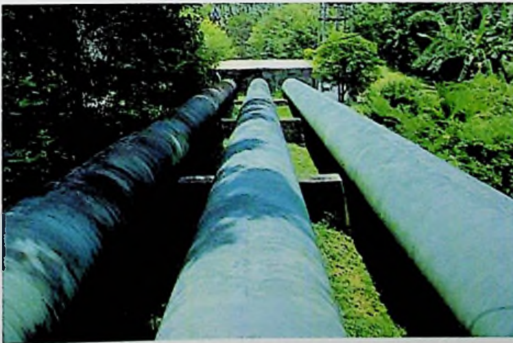
Figure 11: Penstock of the Way Ganga MHP
