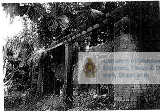
Fig. 46 – Seriously damaged pre-disaster house of T.B. Gunadasa at Kihimbi Ela
