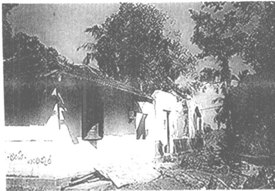
Fig. 40 – Heavily damaged house of H.S.B. Wijethilake at Udahapola, Ginimallagaha
