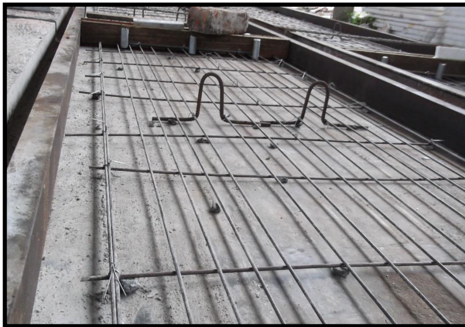
Figure 2-3: Pre-stressed strands of an 85mm thick slab panel (From casting yard at Ekala)
