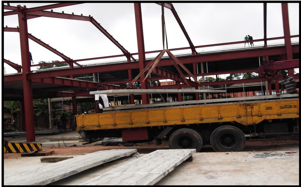
Figure 2-5: Lifting a panel using a crane at a construction site (A photo from the construction of a new hospital building at Negambo Hospital-2015)
