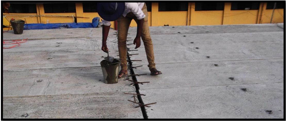
Figure 2-6: The joint between two slab panels is interlocked with pieces of 10mm steel bars (A photo from the construction of a new hospital building at Negambo Hospital-2015)
