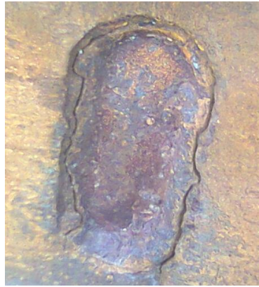
Figure 4: Crack in circle
