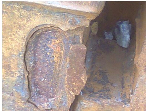
Figure 5: Crack in head
