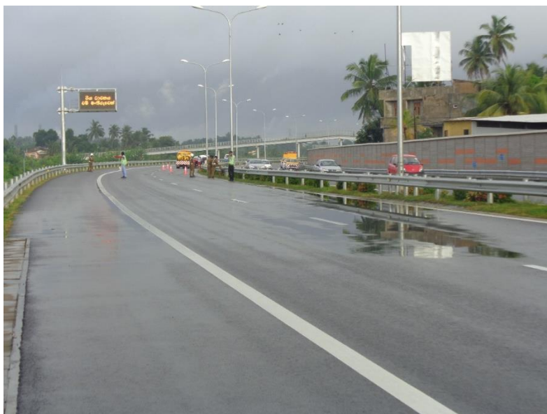
Figure 4-6 Water stagnation after a rain in 7.3 km KD
