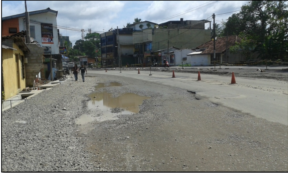
Figure 3-10: Water stagnation at ABC Fill
