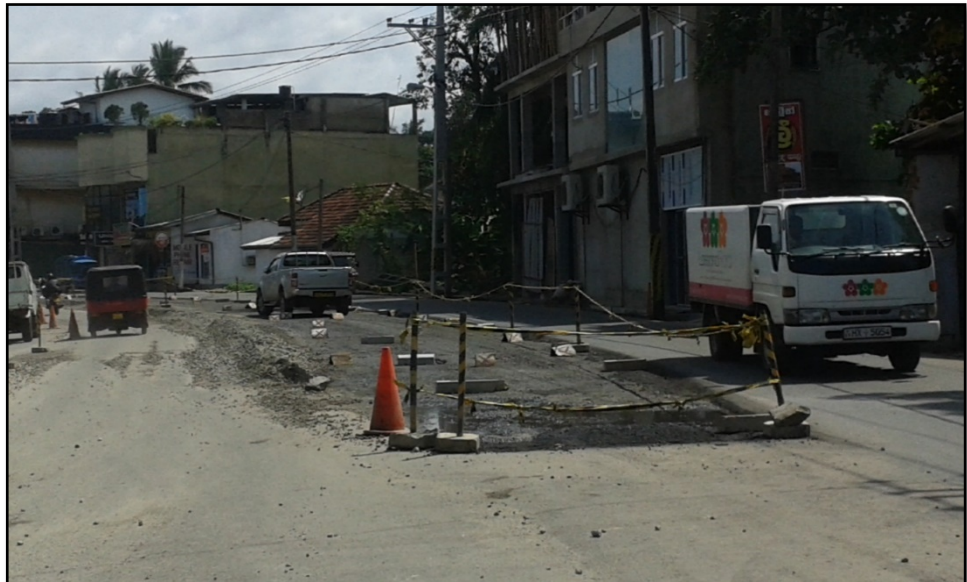
Figure 3-11: Poor Barricading at the middle of the carriageway
