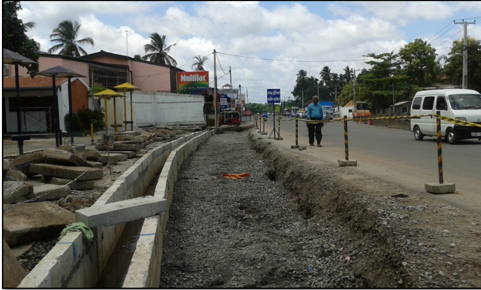
Figure 3-12: No safe passage demarcated for pedestrians
