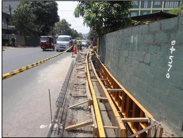
Figure 4-4: No space for the pedestrians at B120 Road Project
