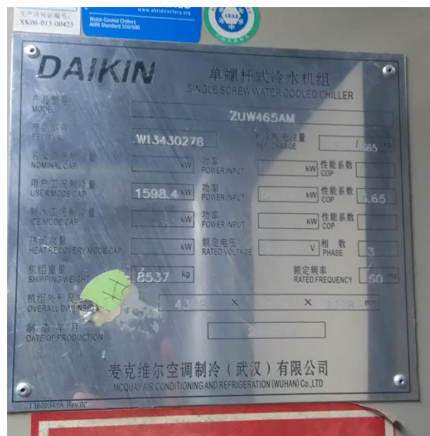
Figure 6: Name Plate Data of Chiller in Cinnamon Lakeside Hotel
