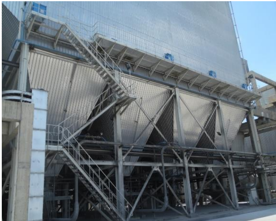
Figure 1.3: ESP units of the power plant
