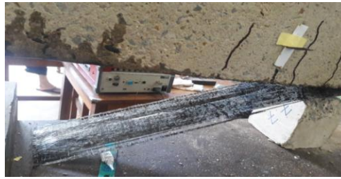
Figure 4.11: Delamination end of CFRP sheet
