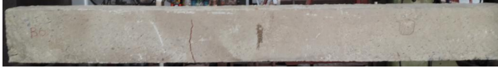
Figure 4.2: Crack patterns in control beams
