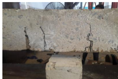
Figure 4.17: Large flexural cracks appeared at the middle of beam
