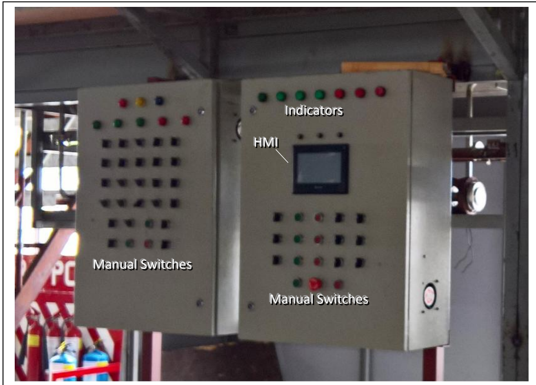
Fig 3.17 Control Panels-Outside View
