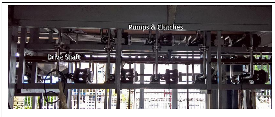
Fig 3.14 Pumps, Clutches and Drive Shaft-View from Front
