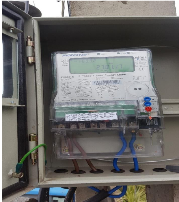
Figure 4.4: Energy meter installed for domestic consumer
