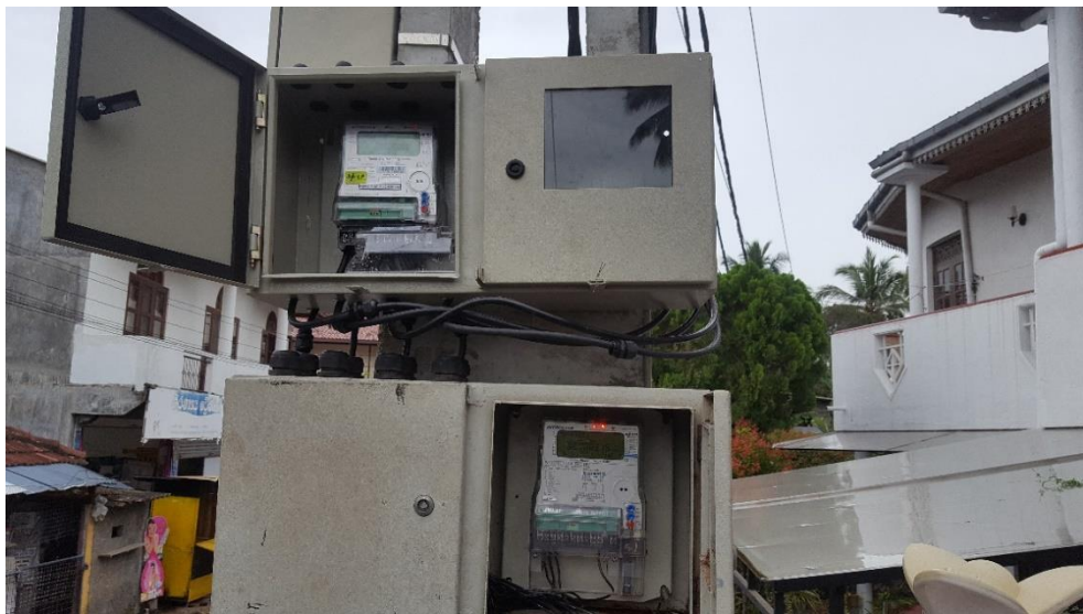
Figure 4.3: Energy meters installed at transformer for source detail collection
