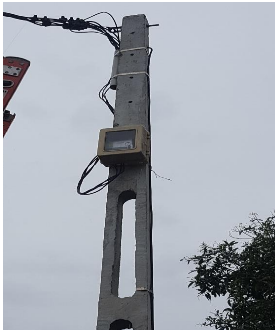
Figure 4.5: Energy meter installed at feeder end
