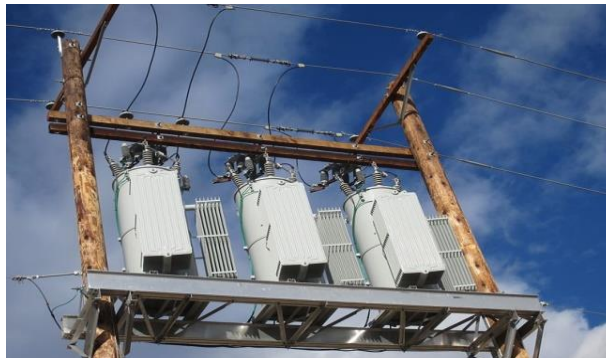
Figure 2:10 Three-phase bank of voltage regulators
