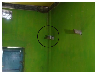
Figure 15, Installed Data Logger in Brick house
