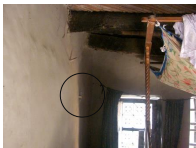
Figure 14, Installed Data Logger in Mud house
