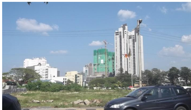
Figure 5.48: Old warehouses in front of the water body being demolished and the lands to be reused for hi-end developments, Source: Author
