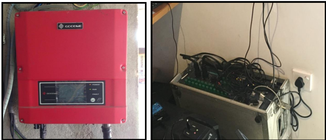
Figure 1 a) GOODWE Inverter b) LEM Power Quality Analyzer
