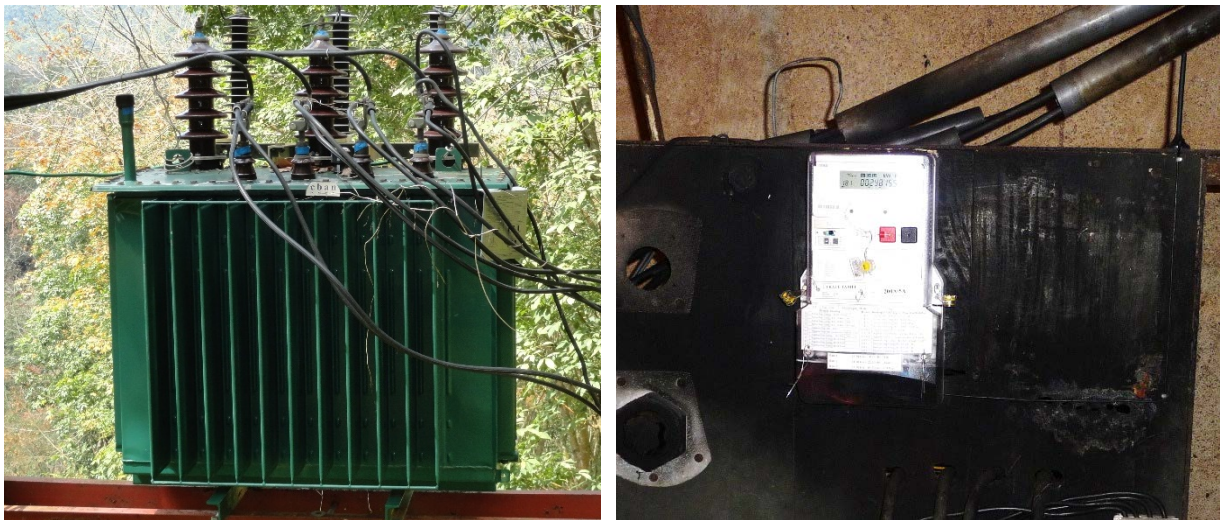
Figure 2.2: Burnt Transformer and damaged wiring and structure at Ukuwelakanda PDS, Horana
