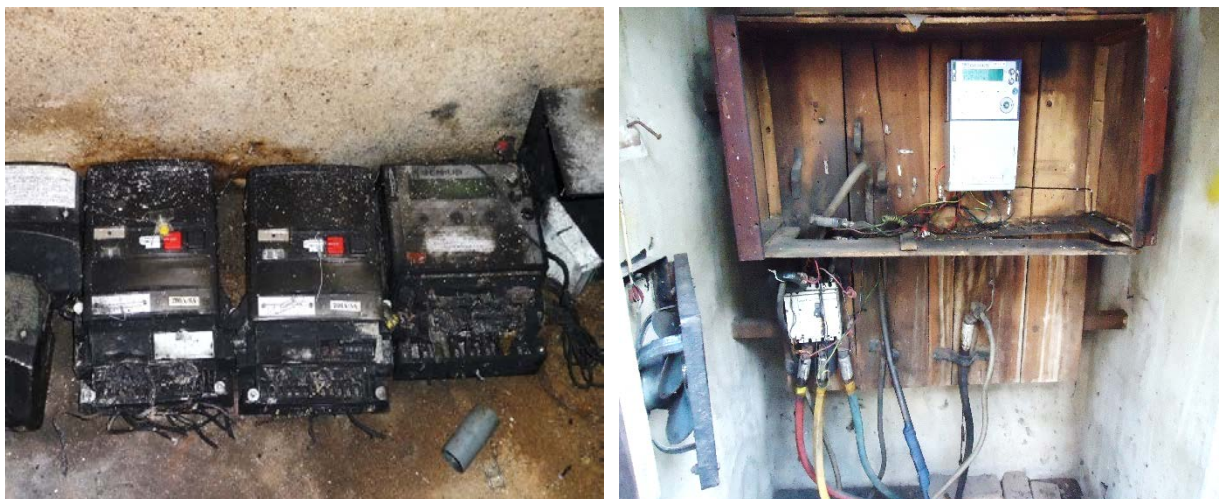
Figure 2.3: Burnt energy meters and damaged MCB and structure at Super Pack Substation, Sri Jayawardanapura
