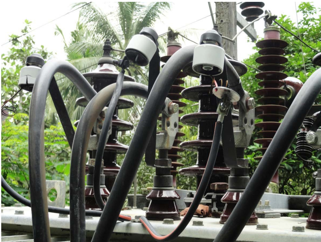
Figure 6.7: Disconnected Arrester at Sripali, Horana
