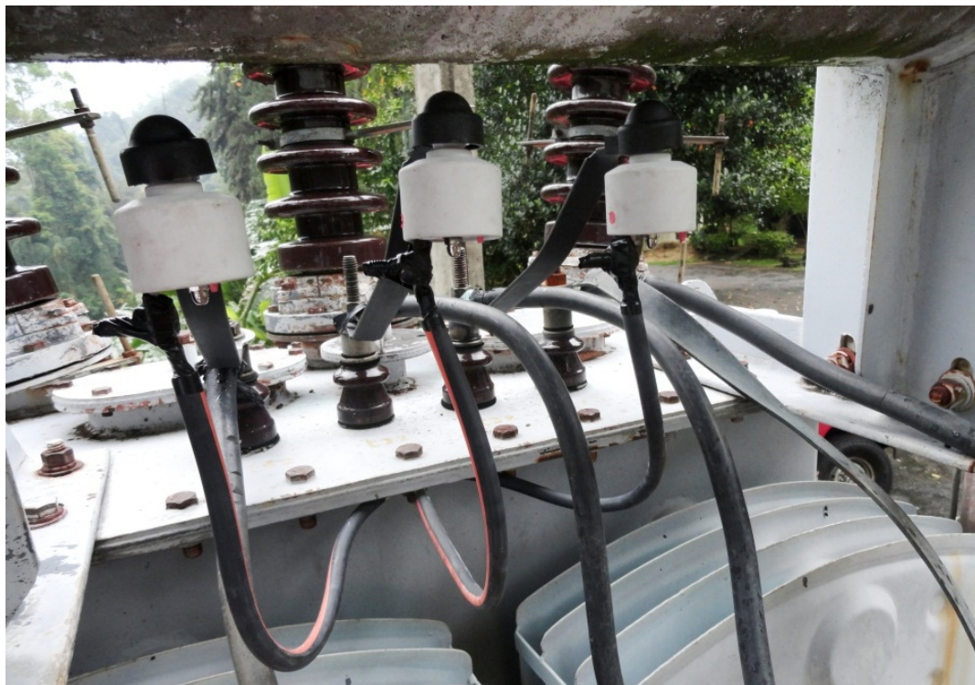
Figure 6.5: Installation at Labugama Water Treatment Plant, Awissawella
