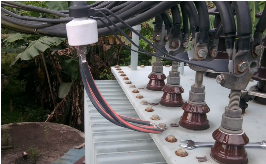
Figure 6.4: LV Arrester Installation at Tea Small Holdings, Horana
