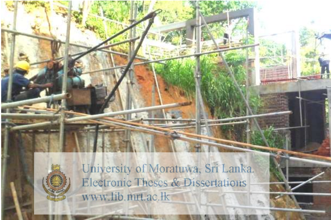
Figure 3.5 GI pipes connected to each other to form a grid both parallel to the ground and the soil nailing surface
