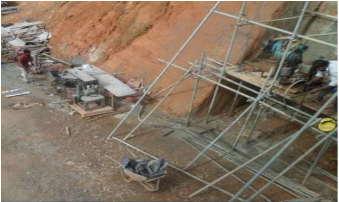
Figure 3.10 - Grouting machine placed on the platform University of Moratuwa, Sri Lanka. Electronic Theses & Dissertations www.lib.mrt.ac.lk
