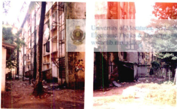
Figure: 3.31 The state of poor maintenance
