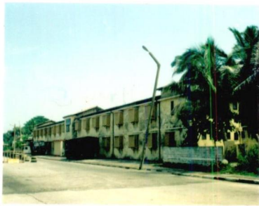
Fig: 71 The abandoned buildings along the landside boundary.
