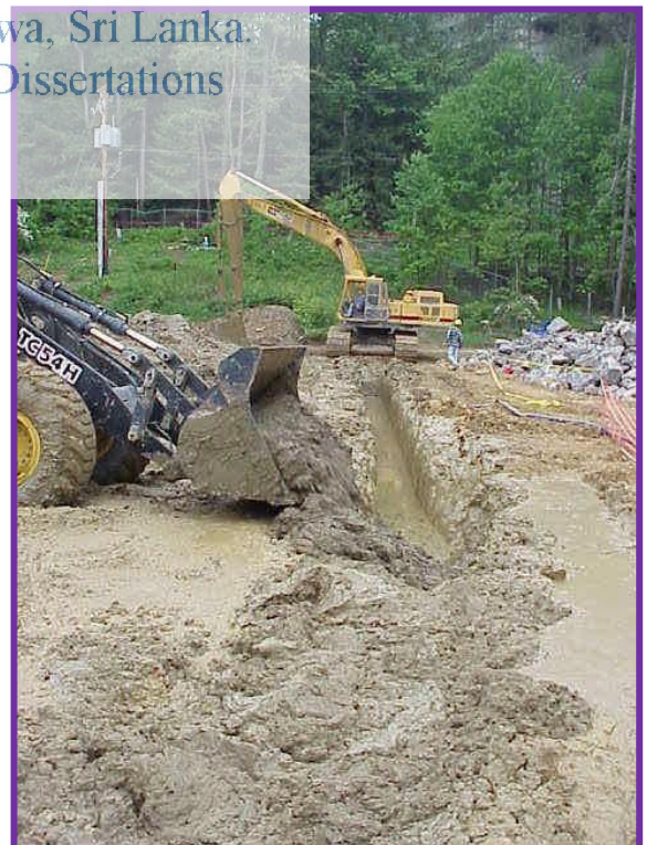
Figure 2.7 – Slumping down the backfill
