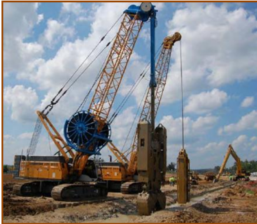
Figure 2.17 - Photograph of Clamshells (foreground) and Long Stick Excavator (background) excavating the Smithland Cutoff Wall
