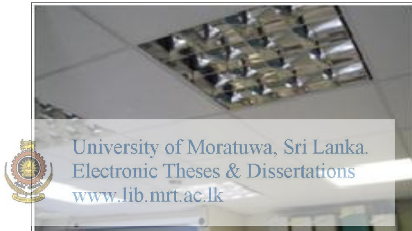
Figure 2.4: Inappropriate luminaries for application modular lay-in in industry[7]
