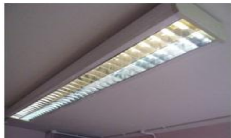
Figure 2.5: Poor maintenance illustrated by mixture of lamps in luminaire [7]
