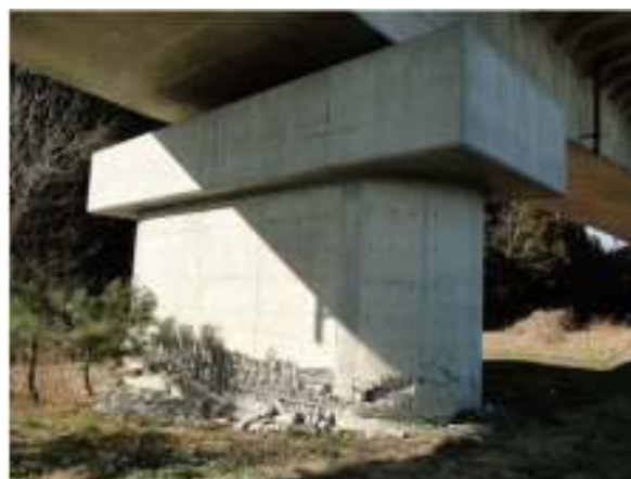
Figure 2-9 Pier failure due to base shear [13]
