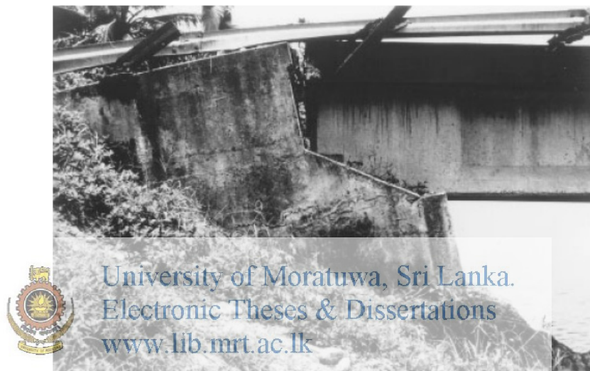
Figure 2-10 Abutment failure due to liquefaction[12]
