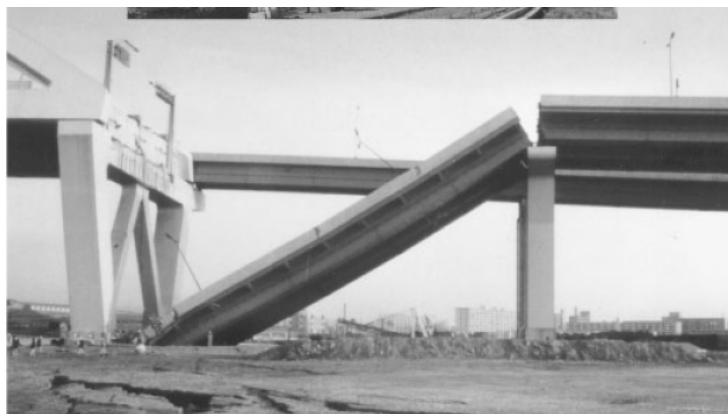
Figure 2-7Superstructure dislocation at expansion joint[12]
