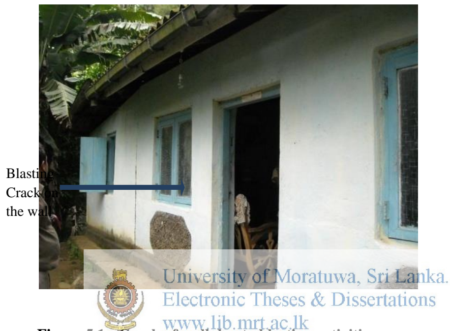
Figure 5.1 - Crack of wall due to blasting activities.
