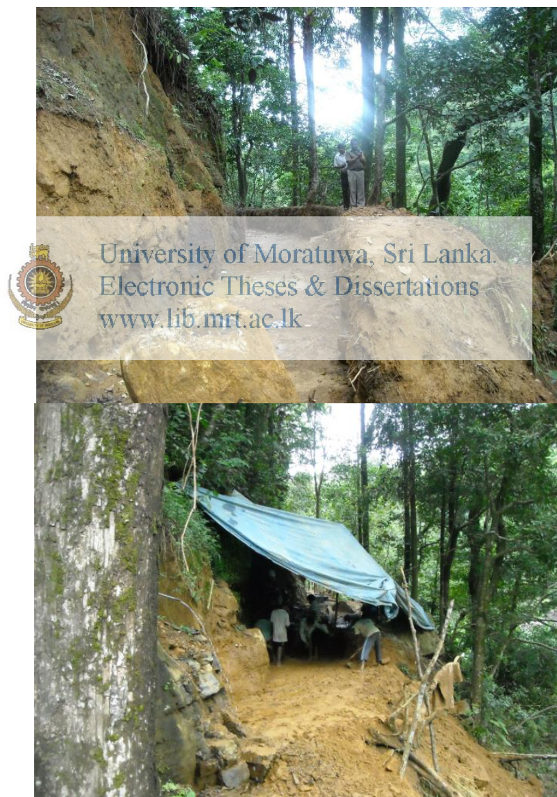
Figure 5.7 - Ground earth surface disturbance and violation conditions
