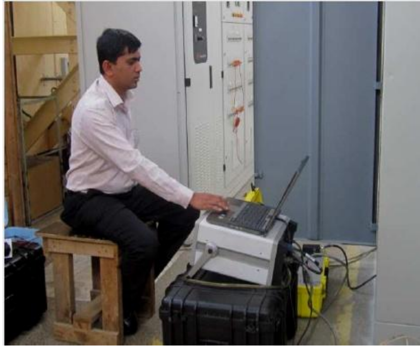
Figure 3.12 : Applying high voltage through the DCR-50 instrument at Wimalasurendra power station 'original in color'
