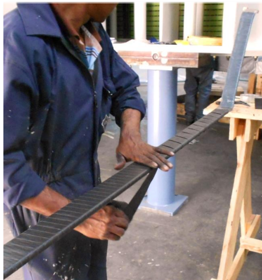
Figure 1.5 : Applying semi-conductive tapes to the roebel bars at New Laxapana 'original in color'
