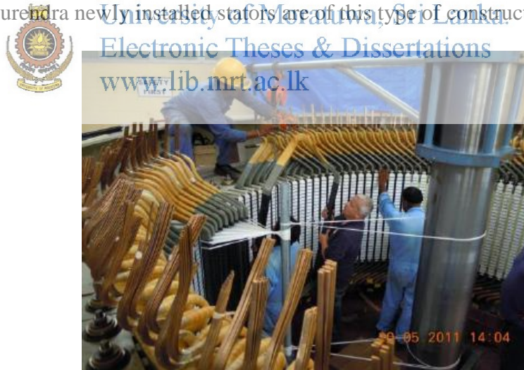
Figure 1.1 : Form wound coils of Wimalasurendra power station ‘original in color’
