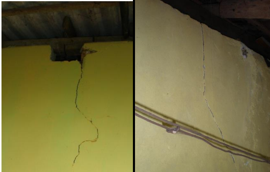
Figure 3.22: wall cracks reported in homes near the Keselhenawa telecommunication tower (Source: Author )
