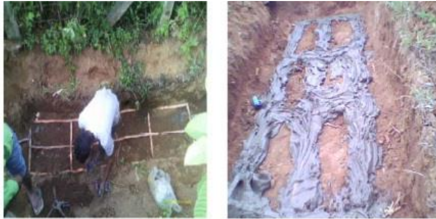
Figure 6.1: Distributed earth with copper earth mesh
