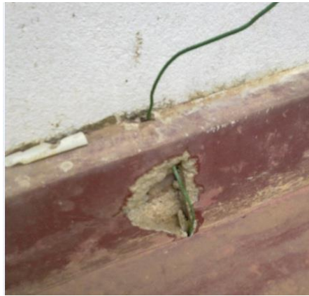
Figure 3.20: wall damages reported in homes near the Madampegama telecommunication tower
