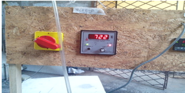
Figure 3.6: Panel of unit
