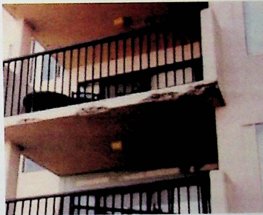
Figure 3.2: Spalling of concrete
