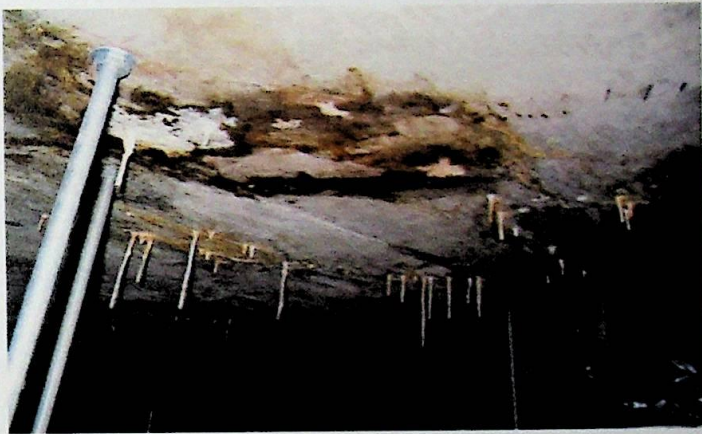
Figure 3.5: Drips along cracks
