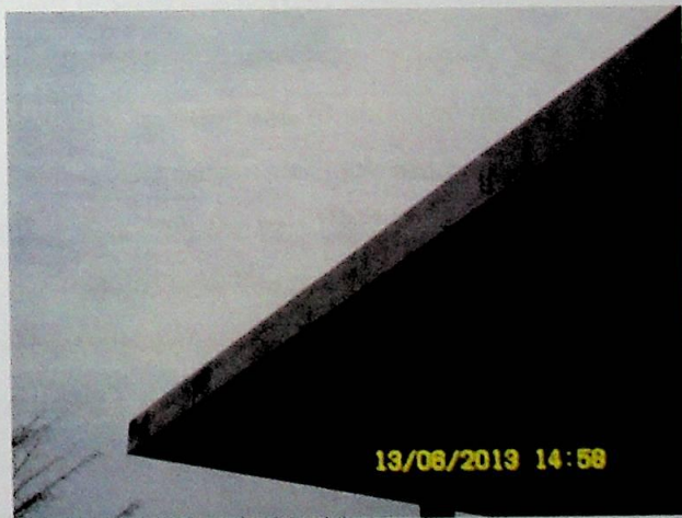
Figure 3.10: Leakages along the edge of the slab
