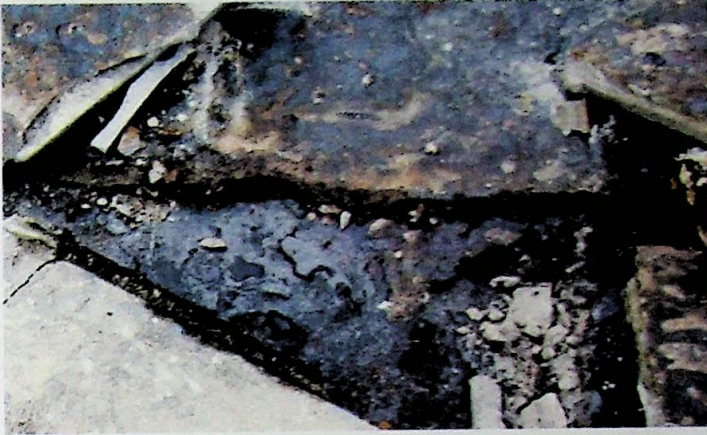
Figure 3.7: Water seepage via loose seam
