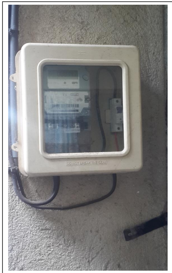
Figure 5.3.1 –Energy meter with Zigbee Module
