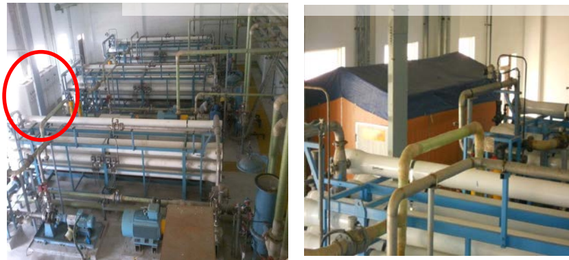
Figure 4.4: Temporary isolation of VSD unit in Desalination plant.
