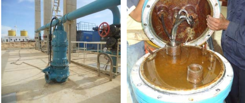
Figure 3.1: Failure of a raw water pump showing water leakage.
