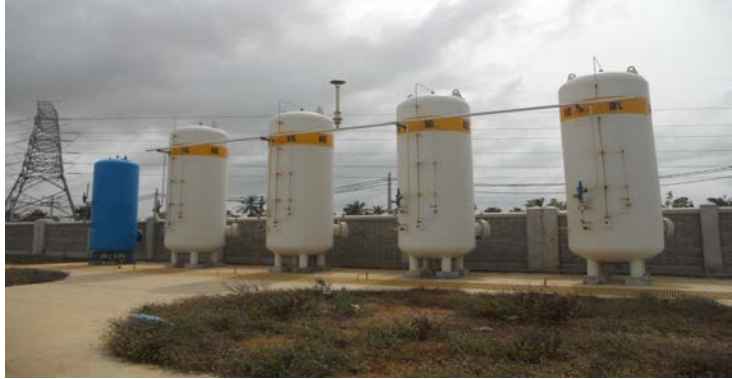
Figure 7.1: Hydrogen storage tanks with the total capacity of 4 x 250 m 3
