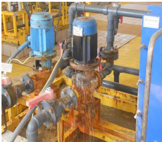
Figure 6.3: water leak through mechanical seal.
