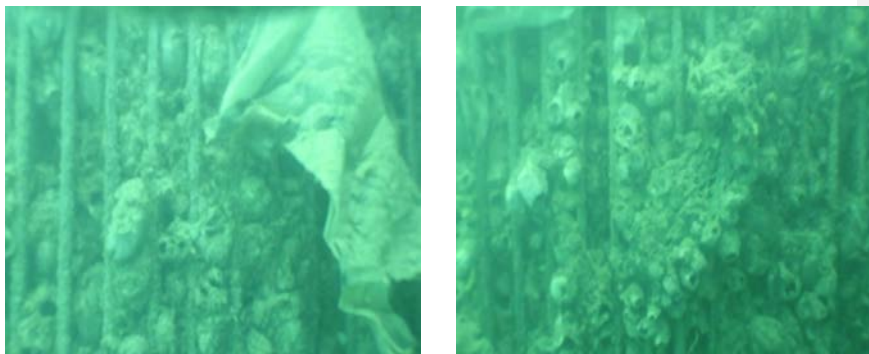
Figure 6.5: Barnacles growth in bar screen due to lack of dosing of NaOCl .
