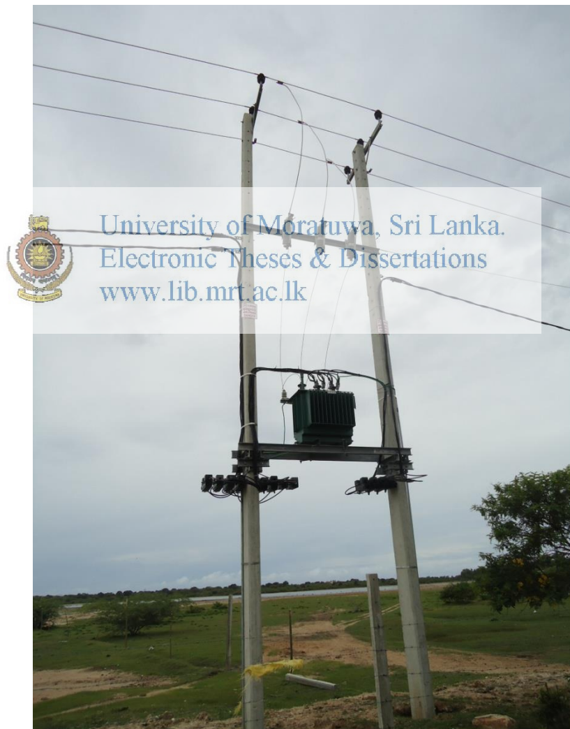
Figure 3.1: Pole mounted distribution transformer
